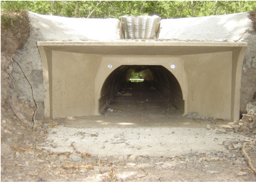
Photo 2: One of the four under-road tunnels installed to allow small vertebrates to safely travel through their habitat. Entrance Road, WLNP
