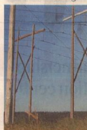
ALtaLink environmental specialist Nikki Kreschko holds up a reflector designed to prevent migrating birds from flying into power lines.
